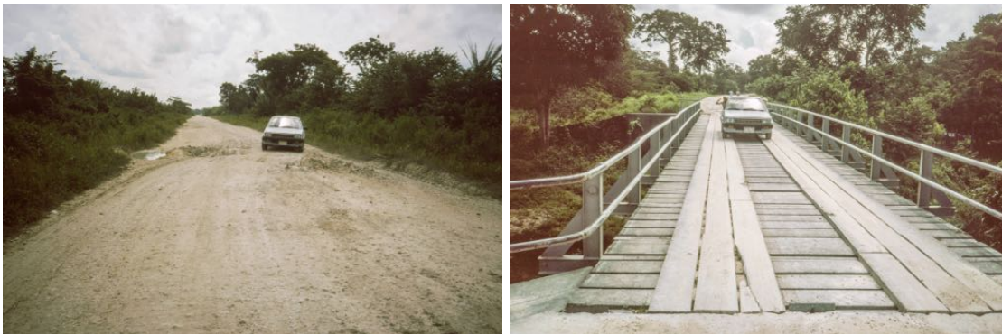
Figure 920. Rutted road and wooden bridge.
