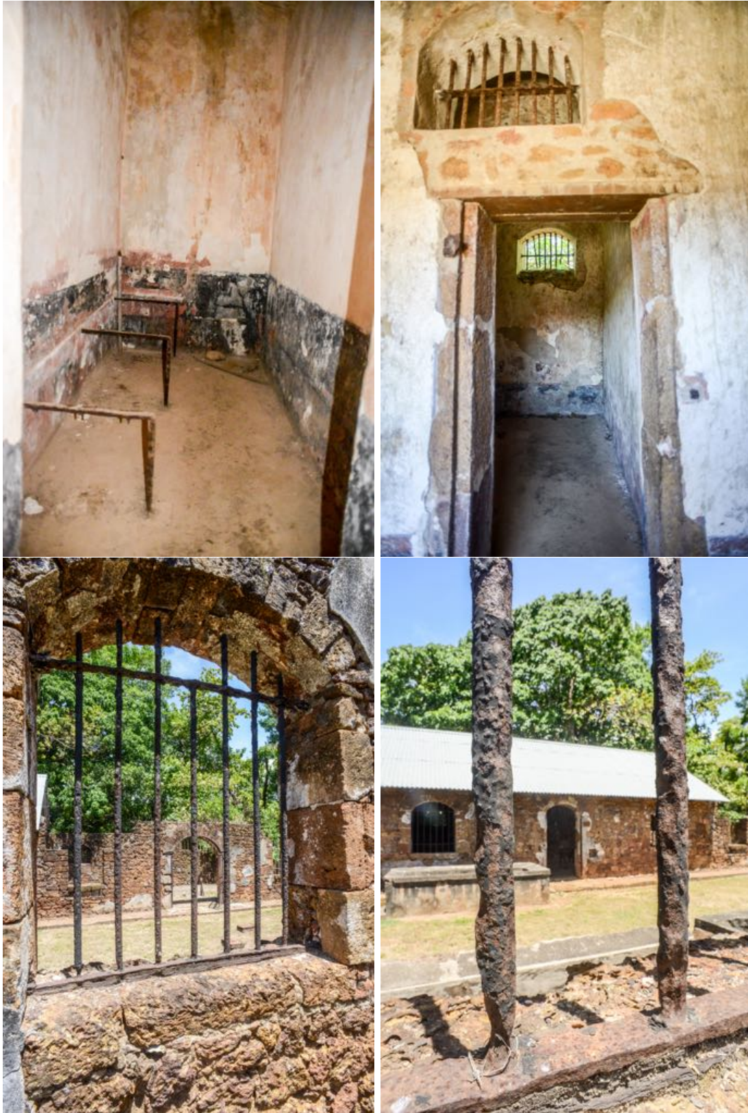
Figure 1050. Cells and rusted iron window bars.
