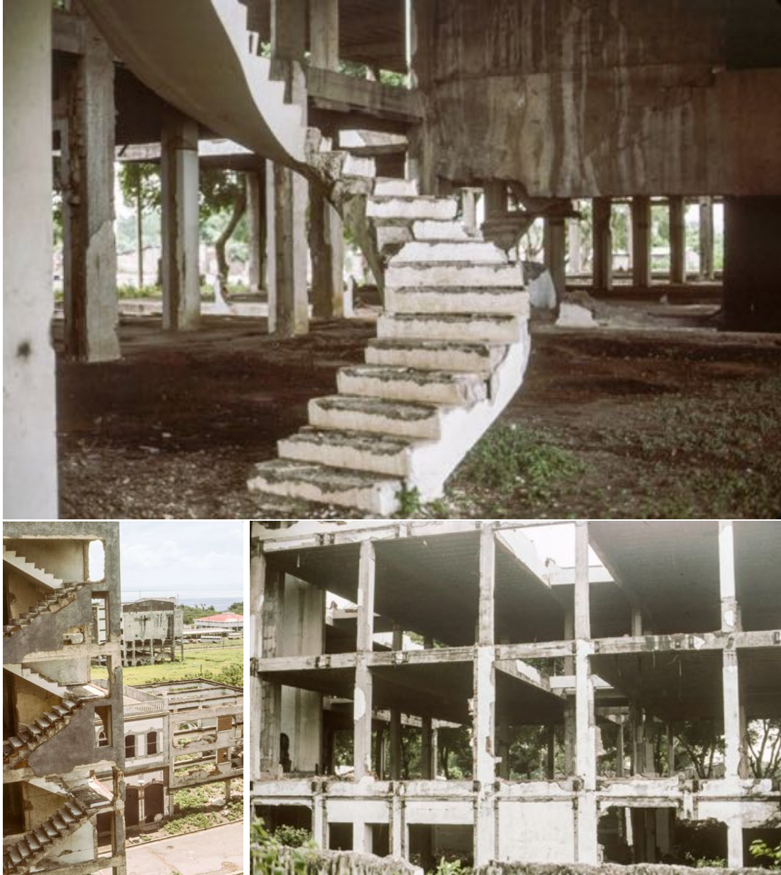
Figure 704. A broken city, 16 years after the earthquake.
