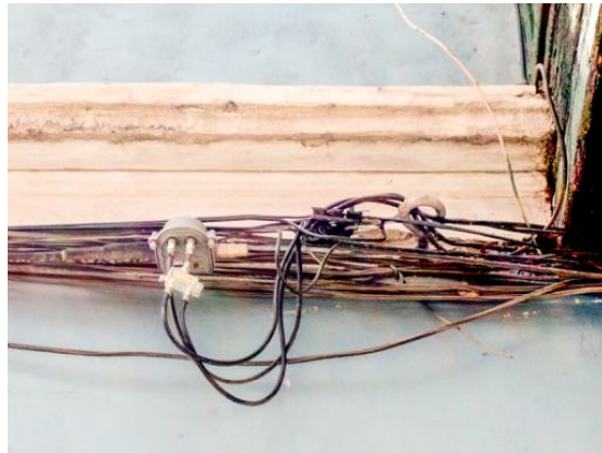
Figure 1158. Open air electrical wiring Bolivian style.
