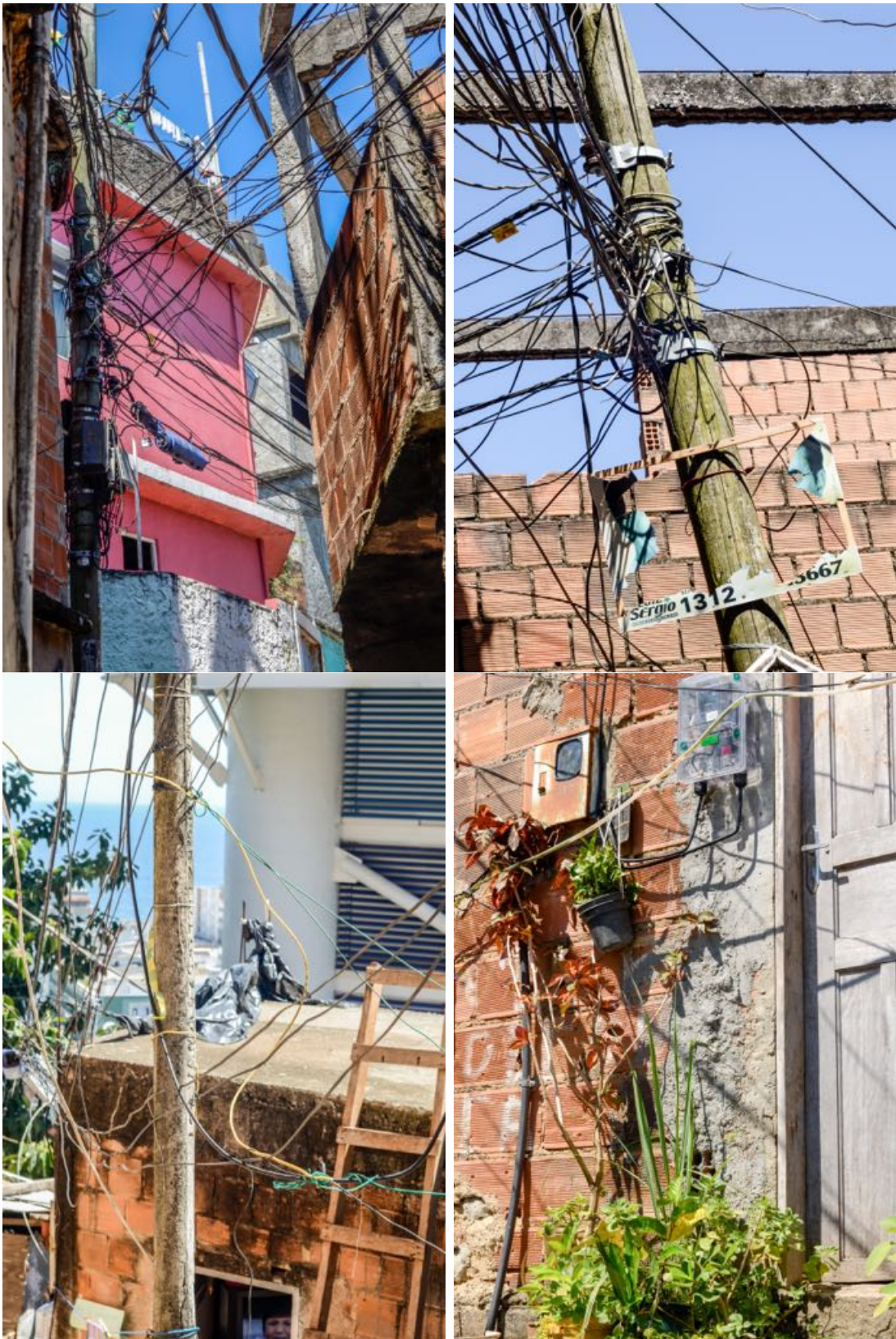
Figure 1496. Makeshift electrical wiring.
